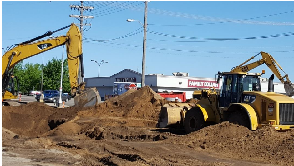
One of many sewer and water infrastructure projects taking place in 2016 in Minnesota. Photo credit: Donald Niles, Wadena, MN
